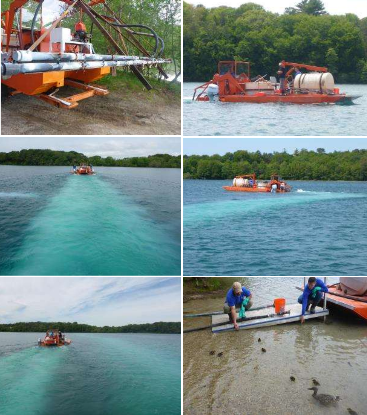
Figure 8. Treatment of Hamblin Pond with aluminum in June 2015
